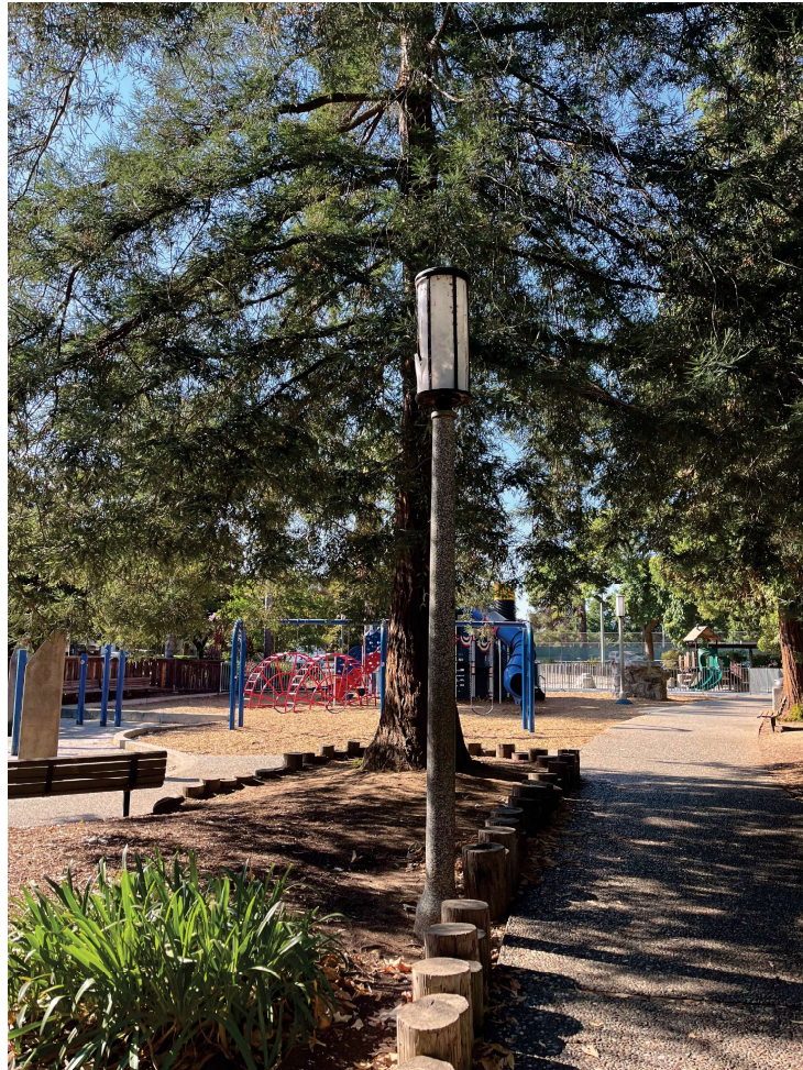
Figure 5: Park's lighting fixture
