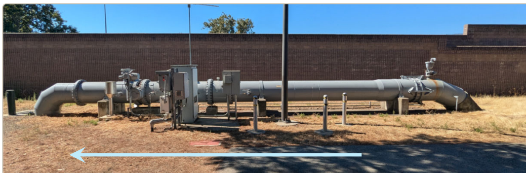
Above: Valley Water Turnout at Wright Ave. Water flows from right (Valley Water's pipes) to left (Sunnyvale's pipes).
