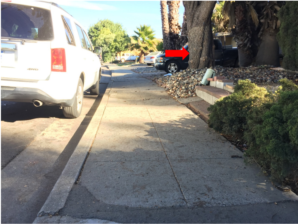
Image #6 – Tree T1, carob (arrow). Sidewalk, curb and gutter cracked and lifted because of enlargement of diameter of several roots. Several previous asphalt repairs are seen.
