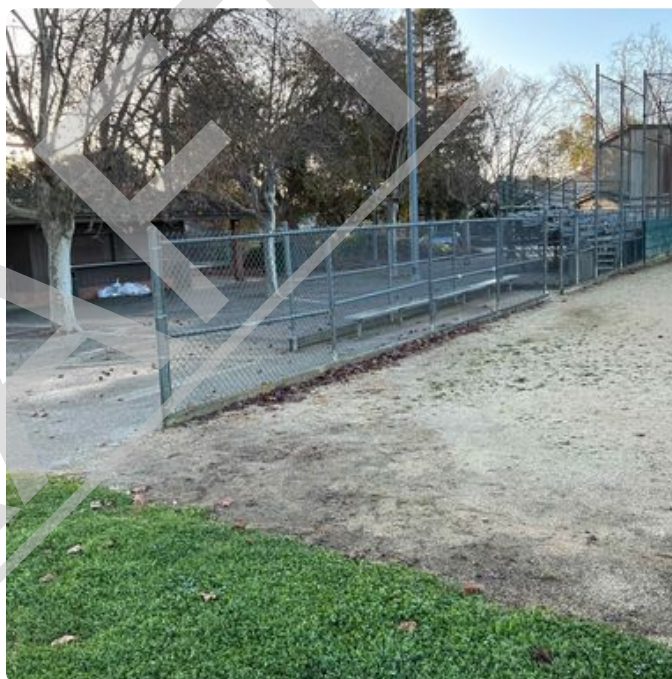
Infield edge needs to be manicured and leveled. Infield does not drain properly. Ortega Park Photos
