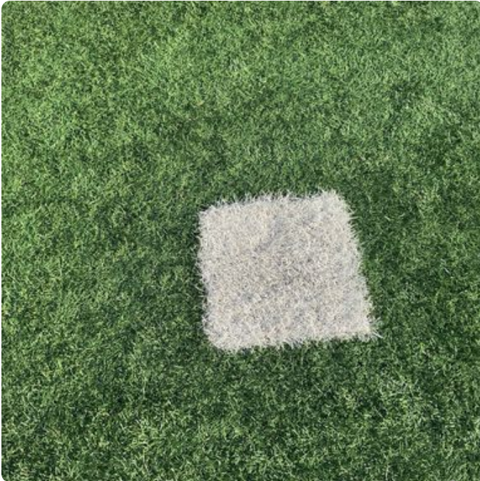
I walked the field, inspecting the seams, the inlaid lines, areas that had evidence of previous repair and I didn't find any area to be unsafe at the time of my observation.
