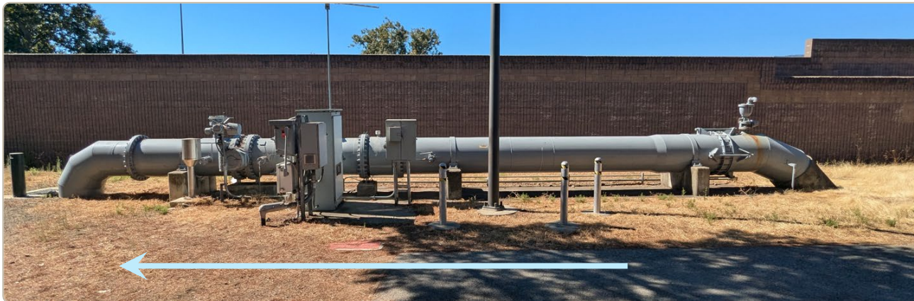
Above: Valley Water Turnout at Wright Ave. Water flows from right (Valley Water's pipes) to left (Sunnyvale's pipes).
