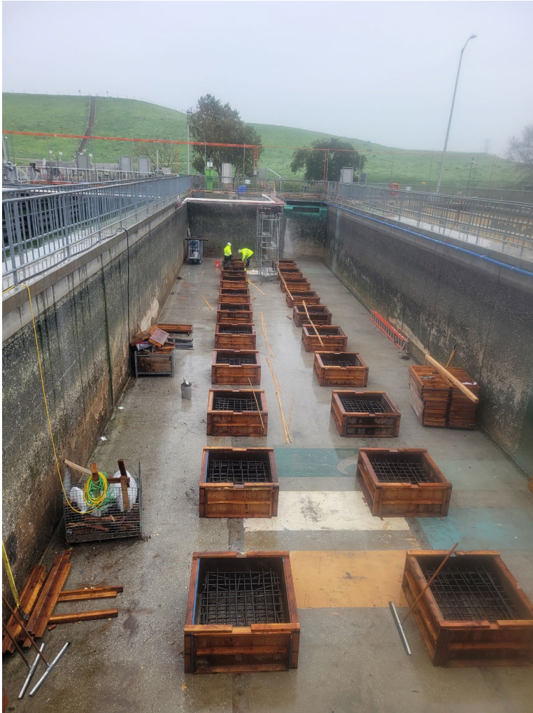
Pedestals for the FRP baffle wall
