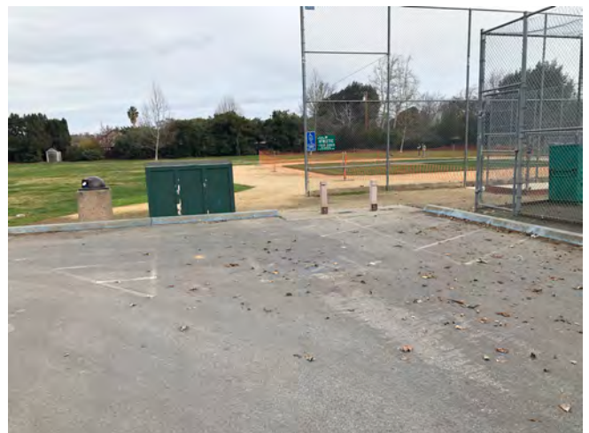
Accessible parking space adjacent to fields requiring improvement
