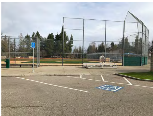
Accessible parking space adjacent to existing cages requiring improvements
