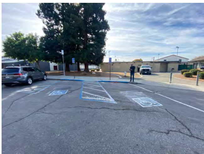
Accessible parking spaces adjacent to pool requiring improvement
