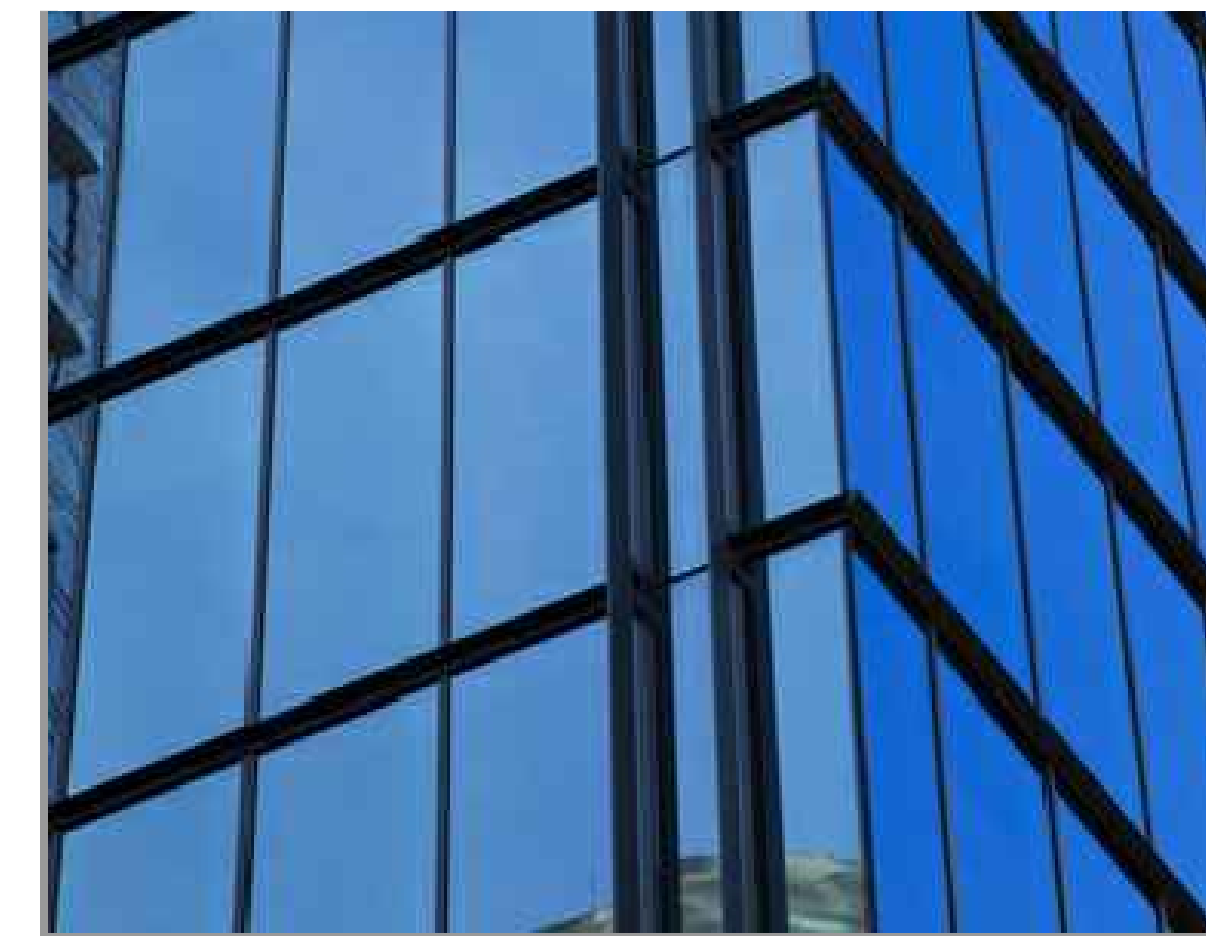
GLZ-1 ENERGY CONTROL GLAZING WITH BLUE TINT AND SLIGHT REFLECTIVE COATING: VIRACON: VE2-M
