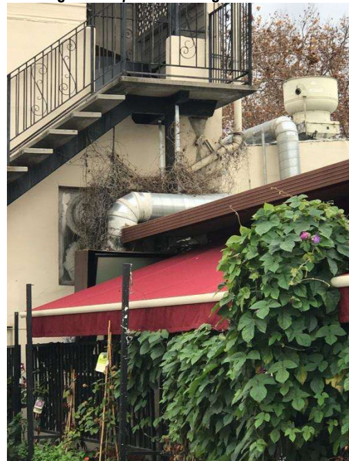
Below: The large, unsightly air ducts and venting at the building rear requires redesign.
