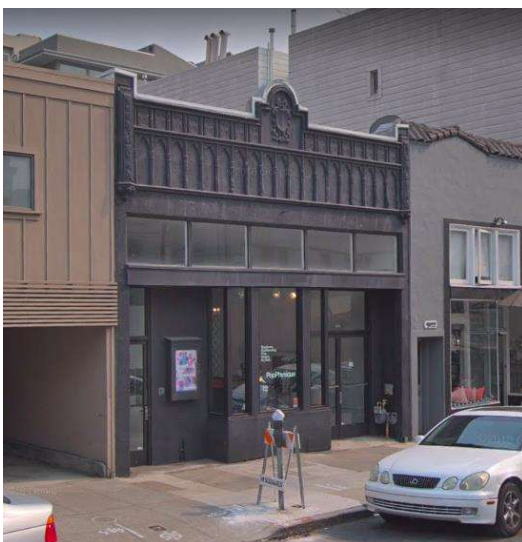
This storefront, which is very intact at the upper level, would benefit from differing colors for trim and at the highly decorative cornice.
