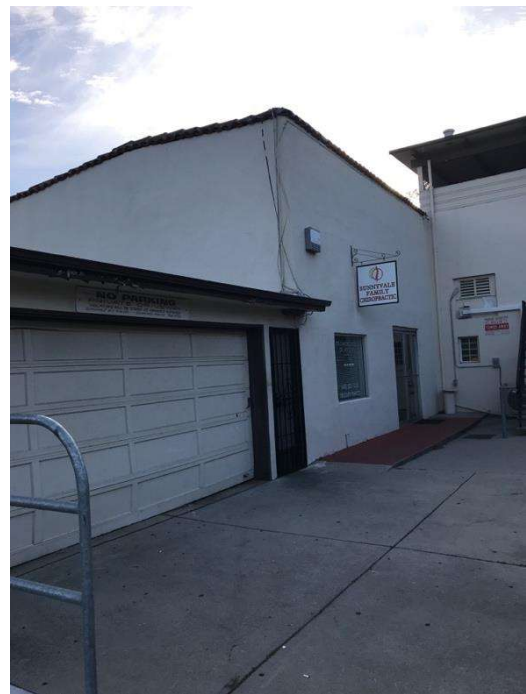
Above: The rear wing and garage are in need of repair, paint and on-going maintenance.
