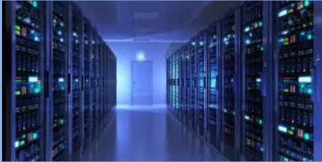
Co-Location Facility (Data Center)
