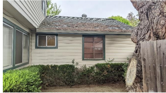
Figure 4. The south facade of the main portion of the building, view north.
