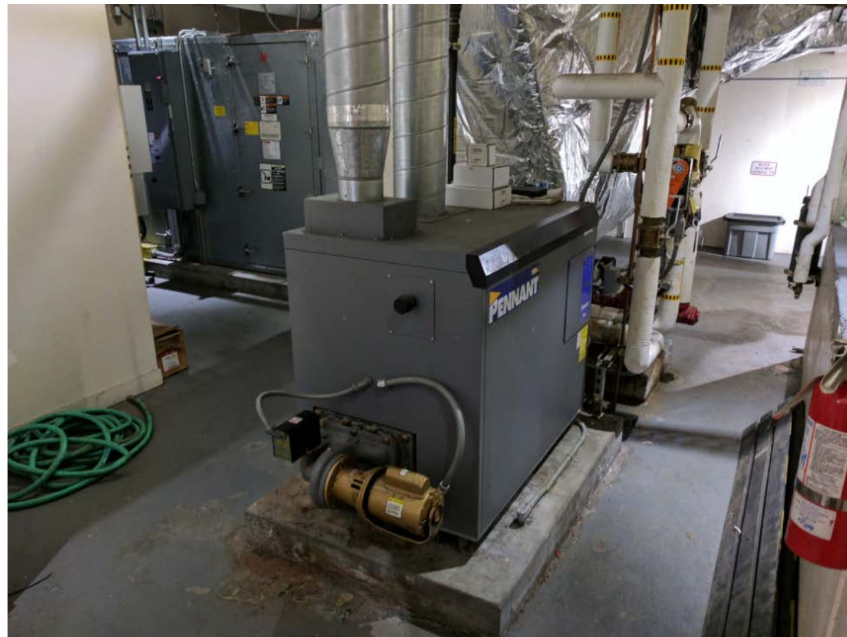
Figure 10: Annex Building Boiler and Multi-Zone AHU
