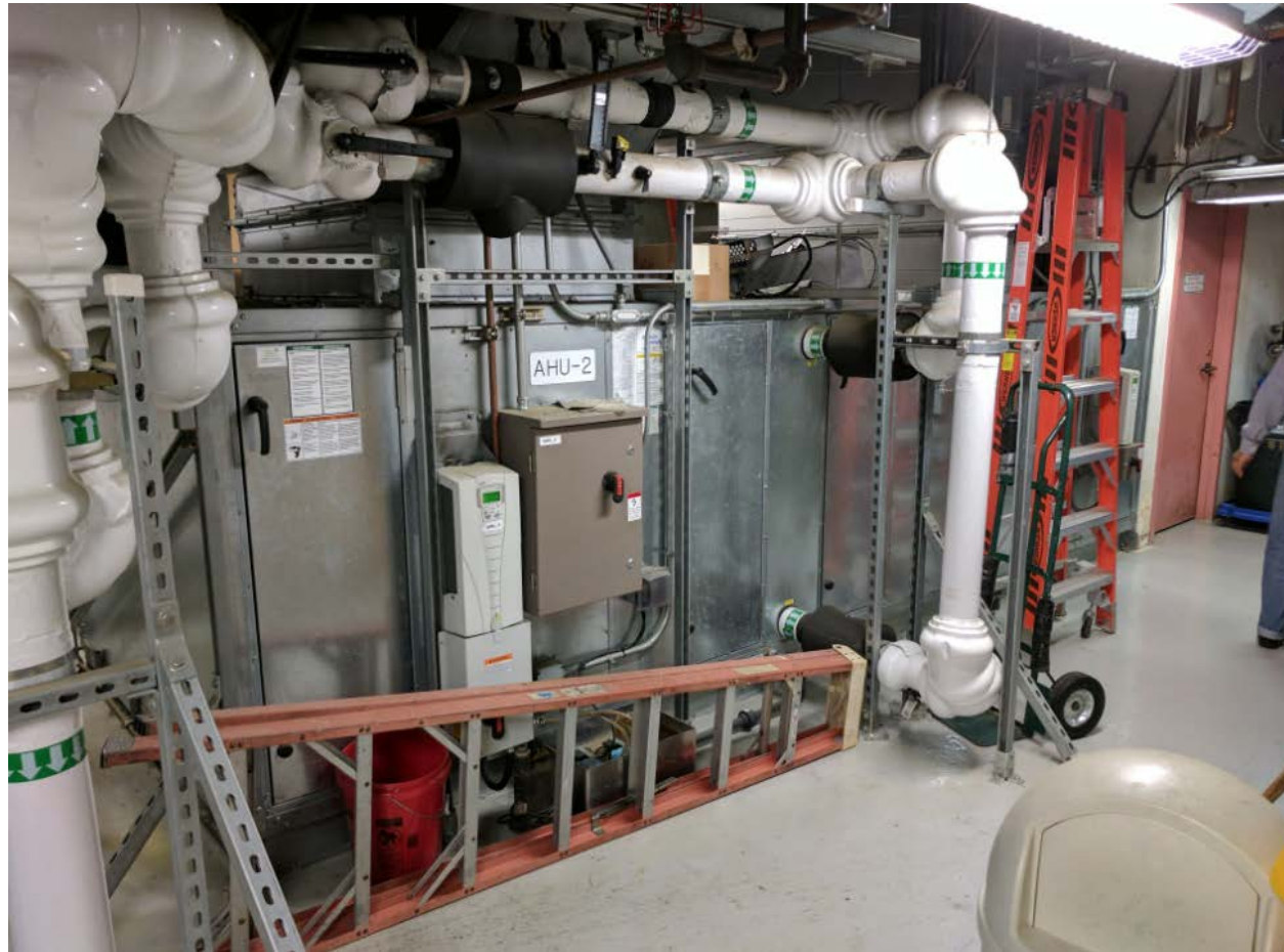
Figure 30: Public Safety Building Air Handling Unit (AHU)
