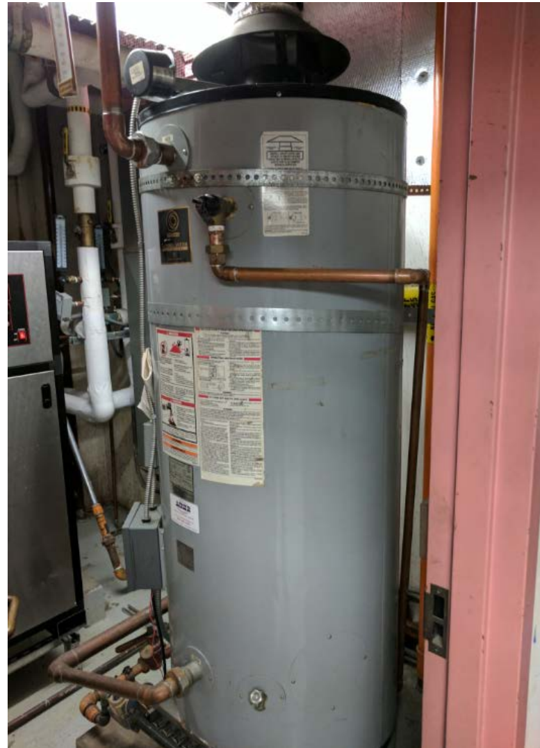
Figure 33: Domestic Hot Water Gas Fired Heater and sewer/storm ejector Pumps
