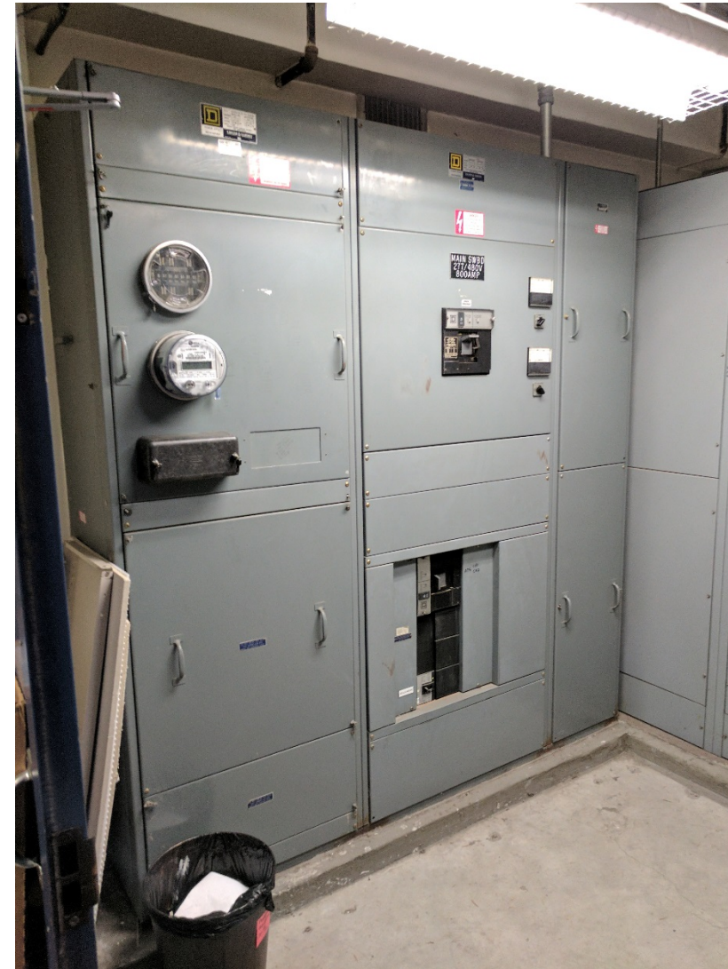
Figure 34: Main Distribution Panel
