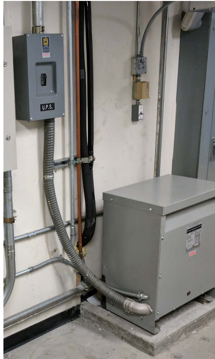
Figure 38: UPS Bypass Panel and Battery Cabinets
