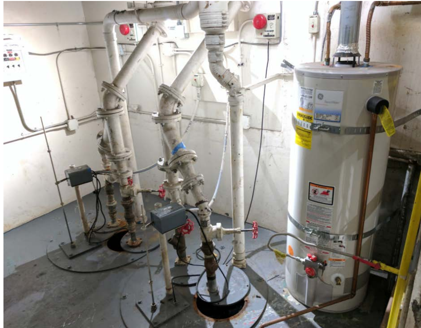
Figure 14: Domestic Hot Water Gas Fired Heater and sewer/storm ejector Pumps
