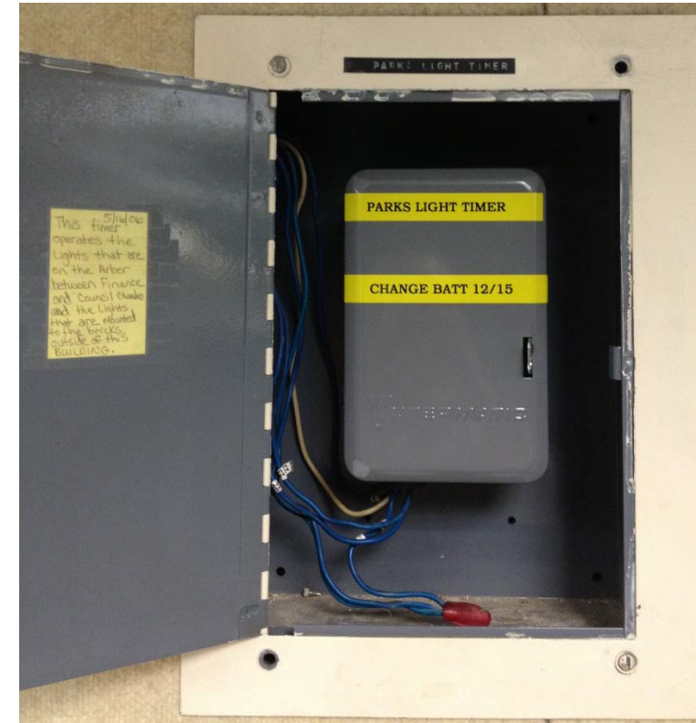
Figure 25: Exterior Lighting Timeclock
