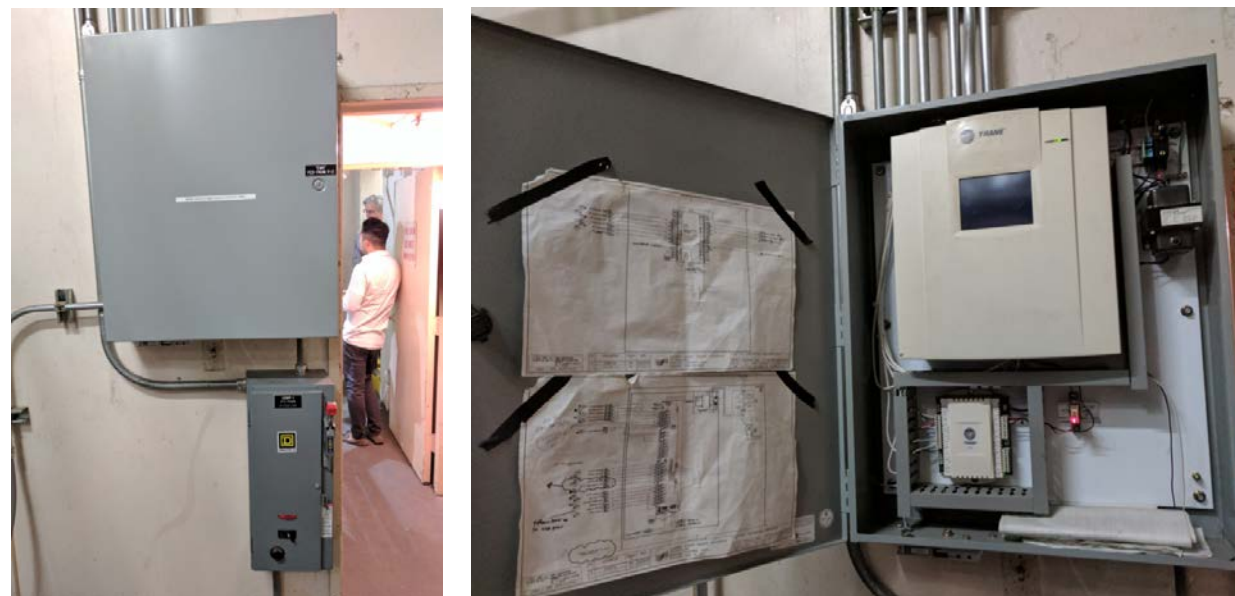
Figure 11: Annex Building HVAC Controls Panel
