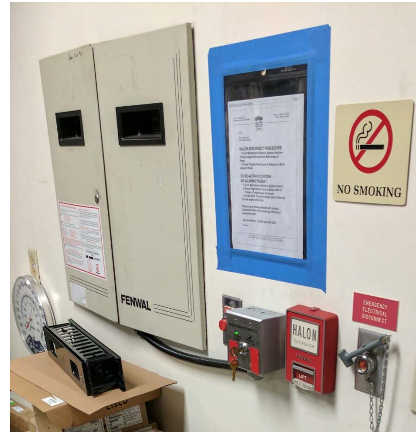
Figure 39: Computer Room Clean Agent Fire Suppression and Raised Floor
