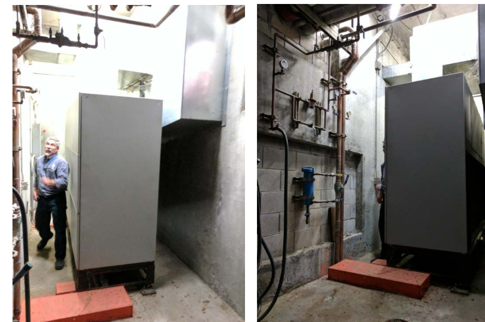
Figure 13: Liebert Air-Cooled Condenser in Areaway
