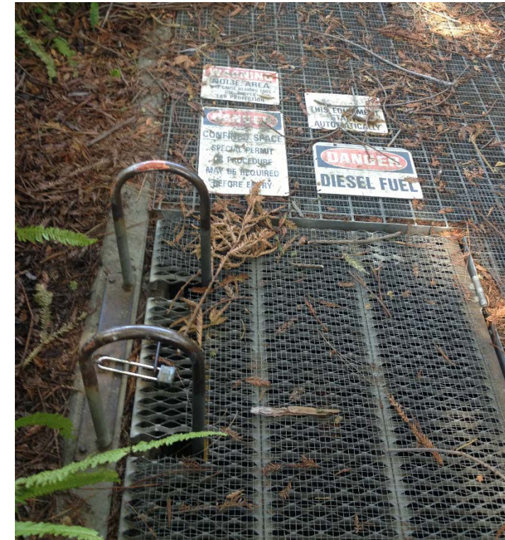
Figure 199: 150kW Generator Pit
