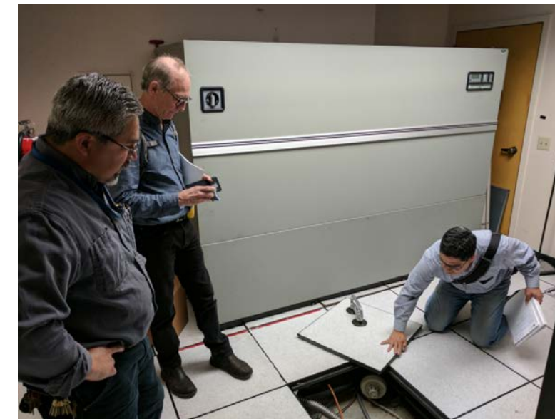
Figure 12: Liebert AC Unit Serving the Data Center
