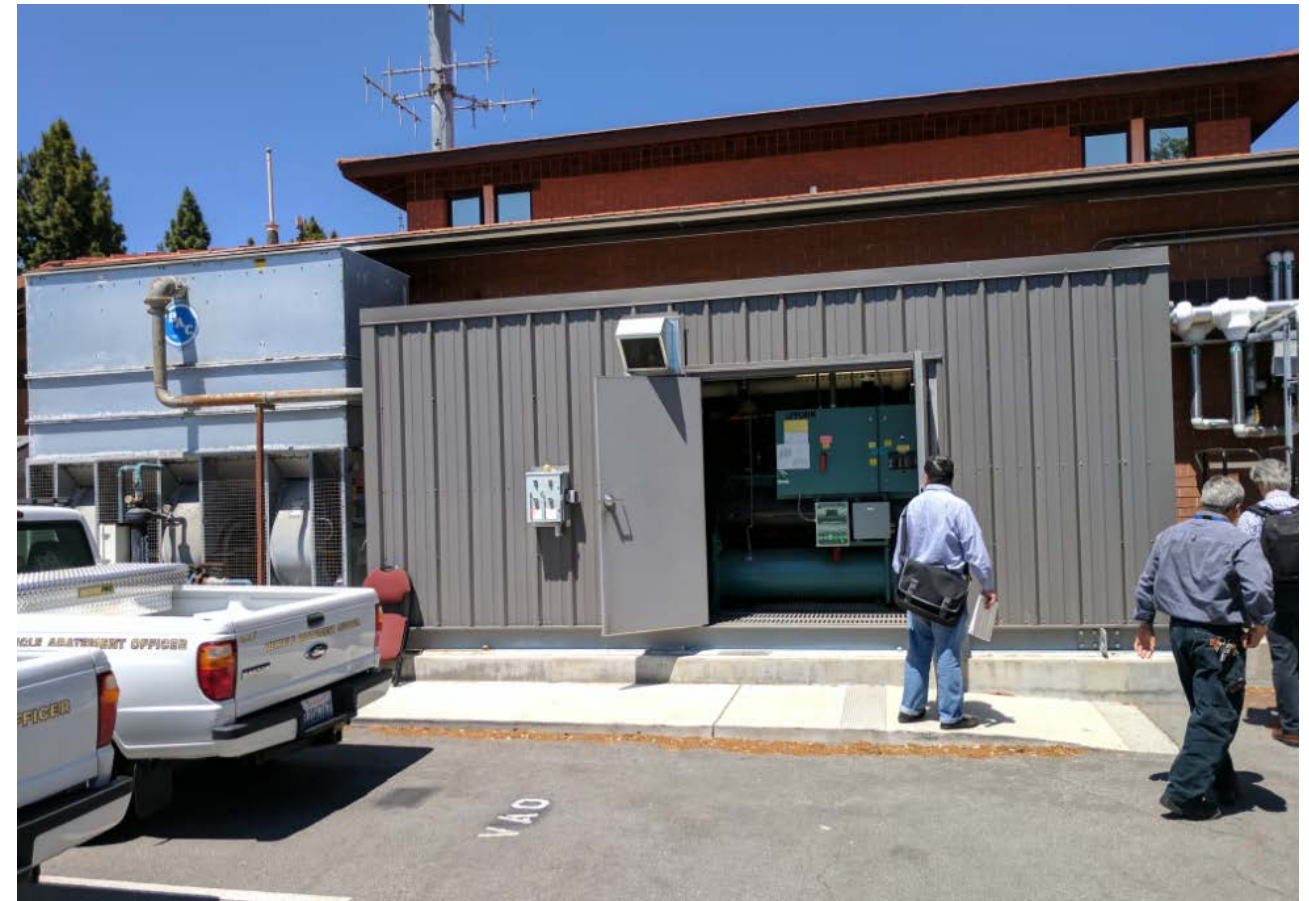
Figure 28: Public Safety Building Cooling Tower and Chiller
