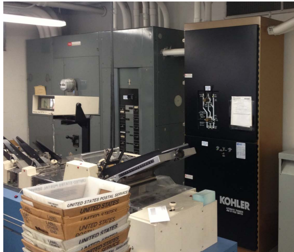
Figure 16: Main Distribution Panel
