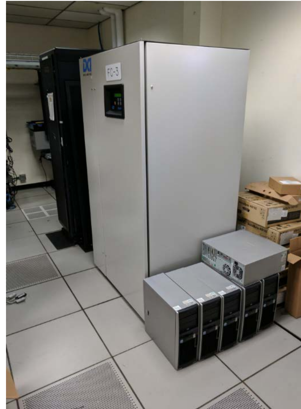
Figure 32: Liebert AC Unit Serving the Data Center
