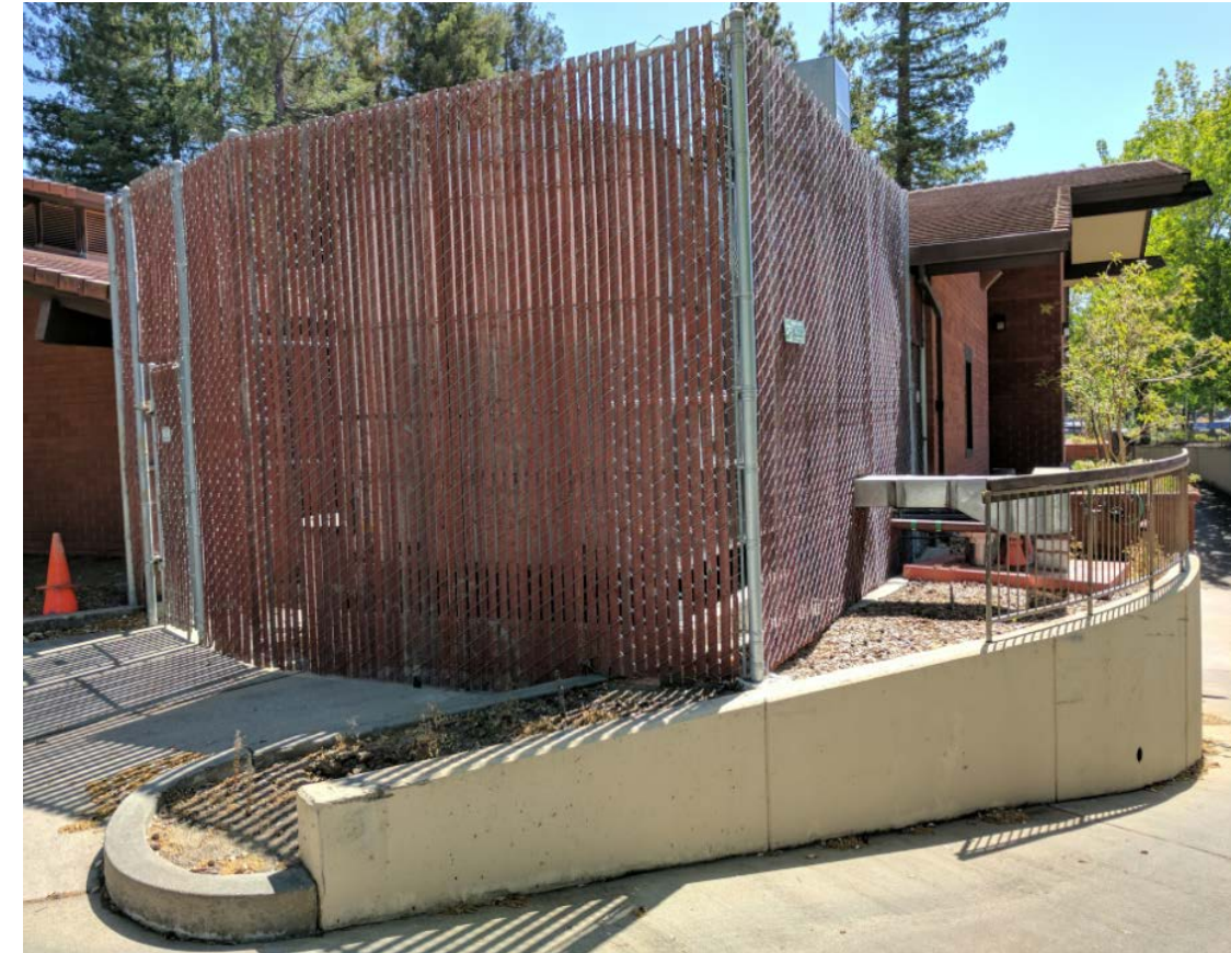
Figure 8: Annex Building Cooling Tower within enclosure
