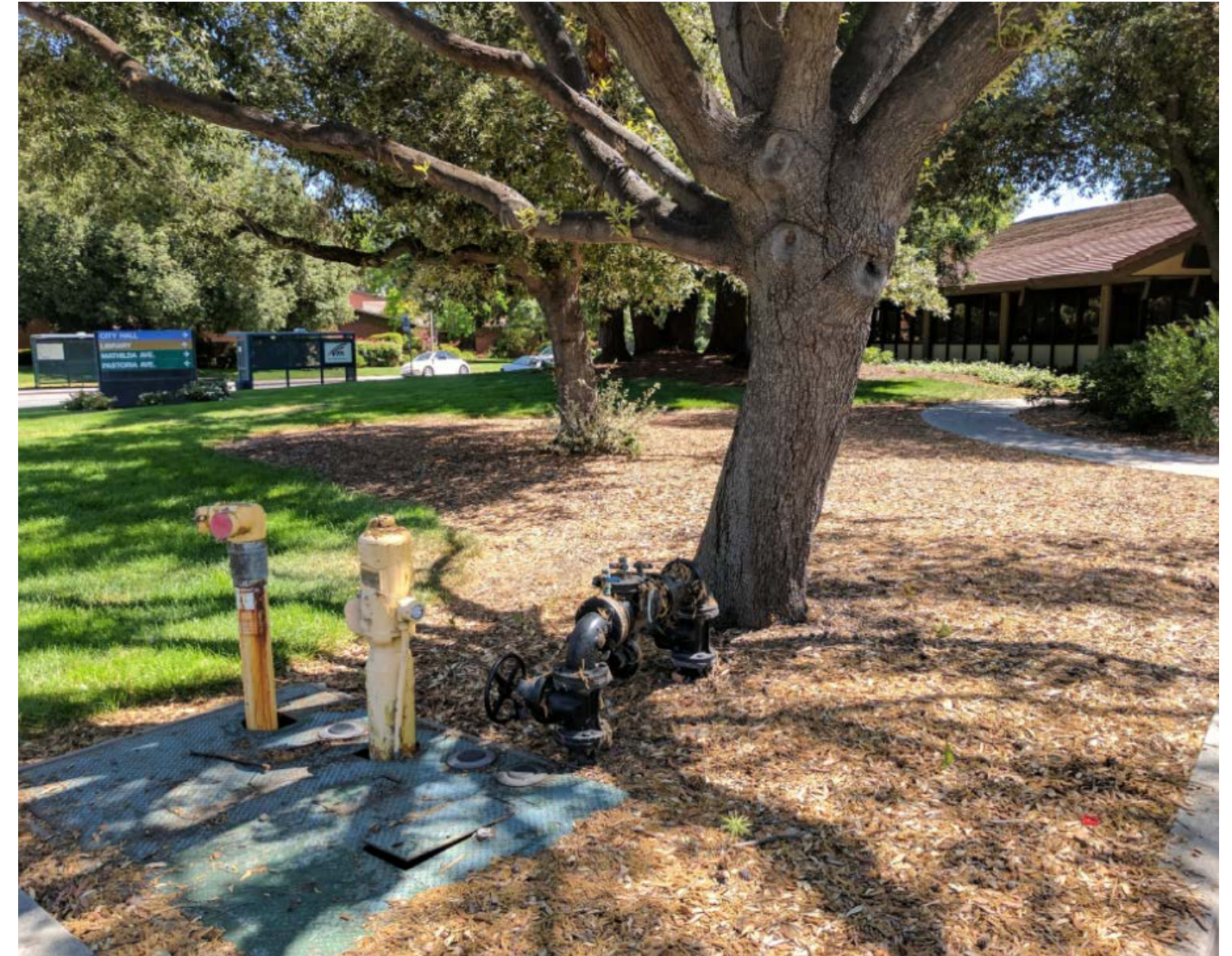
Figure 15: Fire Protection Post Indicator Valve (PIV)
