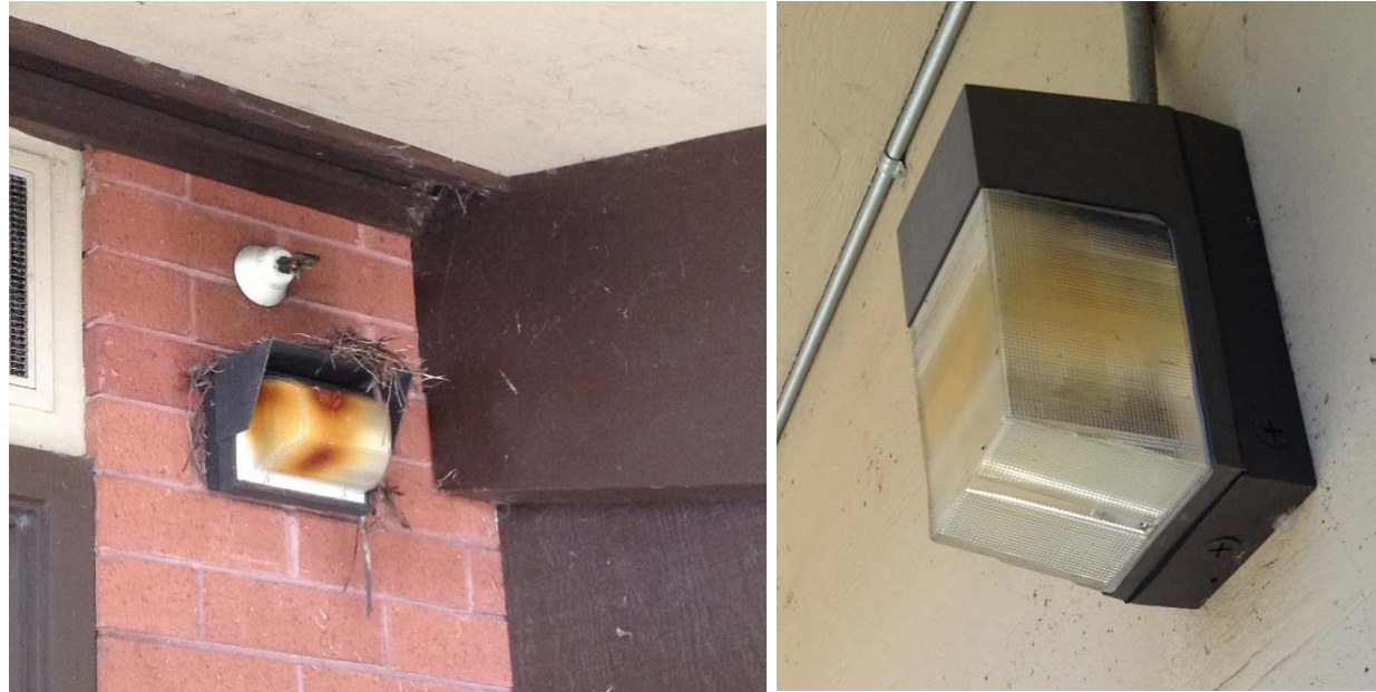
Figure 24: Typical Exterior Light Fixtures
