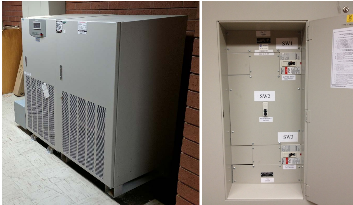
Figure 20: UPS Bypass Panel and Battery Cabinets
