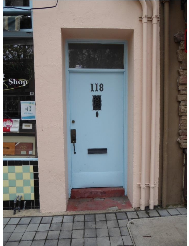
Above: Entry to upper story. Note exposed conduit.
