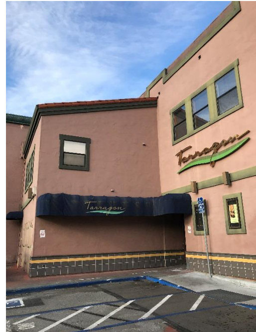
Above: The rear façade has an awkwardly placed awning that should be reconfigured or removed.
