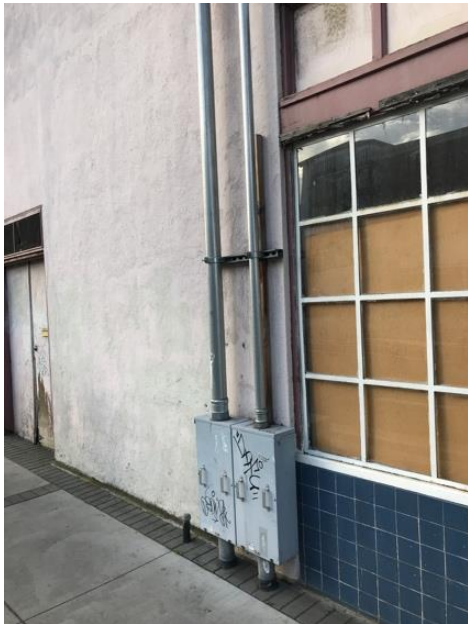
Above: Detail of utility boxes mounted at elevation.
