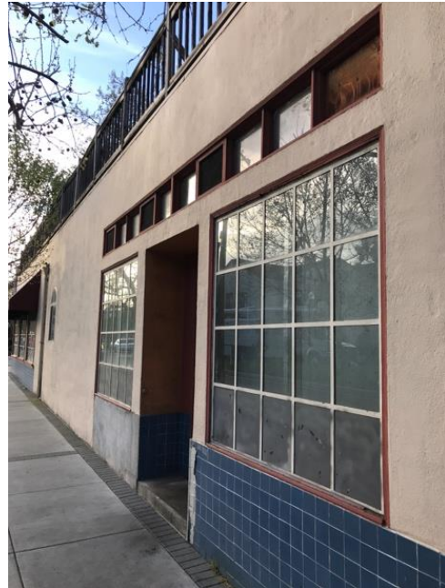
Below: Evelyn Avenue showing missing tile and need for transom window restoration.
