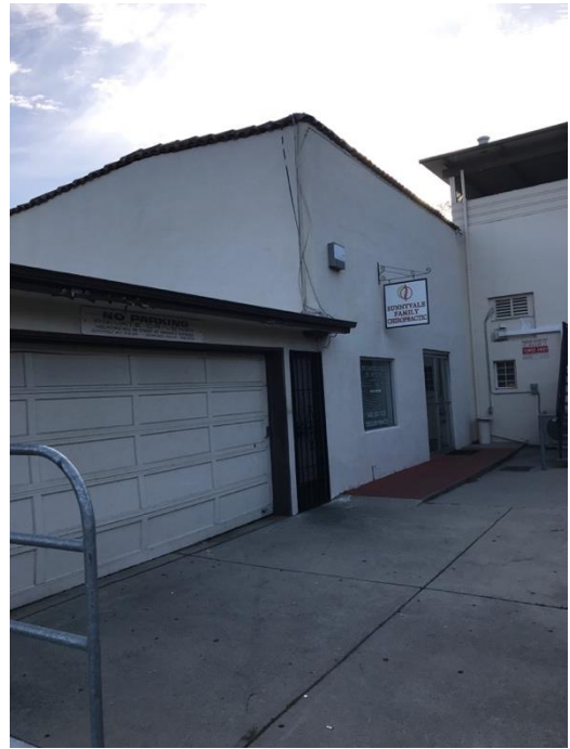
Above: The rear wing and garage are in need of repair, paint and on-going maintenance.
