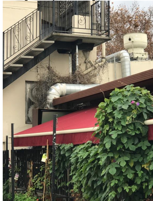
Below: The large, unsightly air ducts and venting at the building rear requires redesign.
