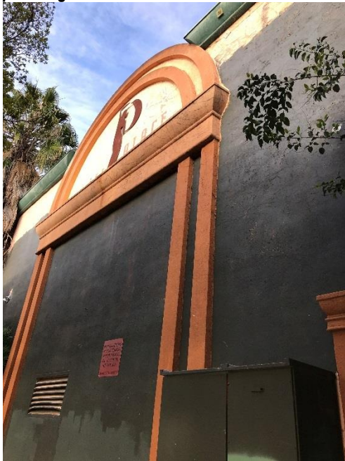
Below: Rear façade showing various paint schemes and patching.
