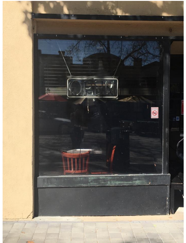
Above: The storefront glazing; note that this building does not have a tile base.
