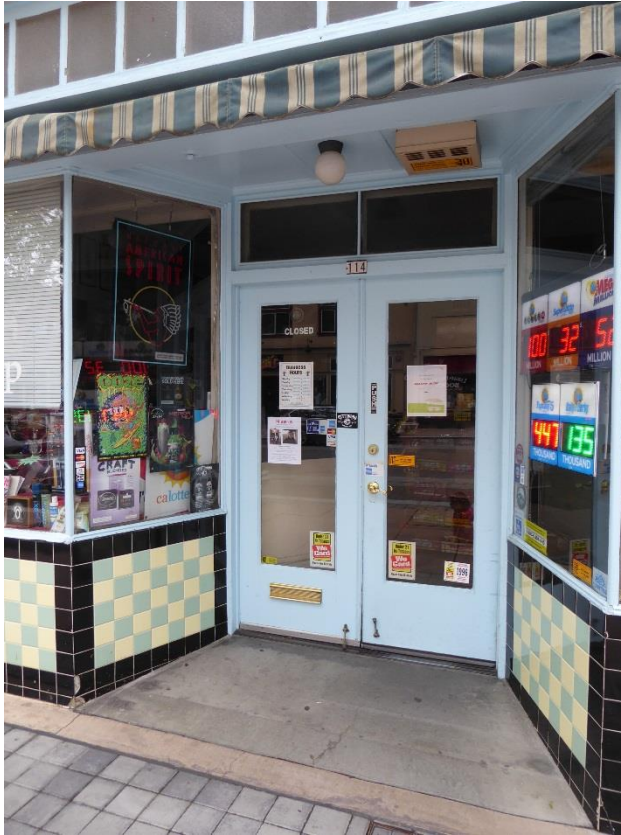
Above: Recessed store entry with original metal storefront windows, multi-colored tile base, and single-panel, glazed, wood double-entry doors with transom above.
