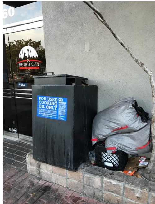
Below: Rear area showing oil storage that should be enclosed.
