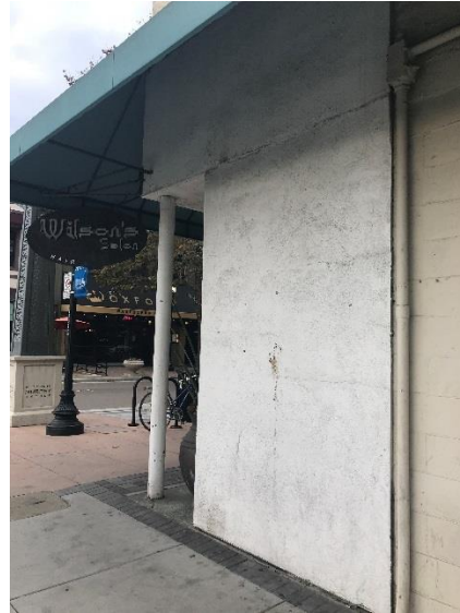
Above: Detail showing corner alteration and incompatible materials and placement.
