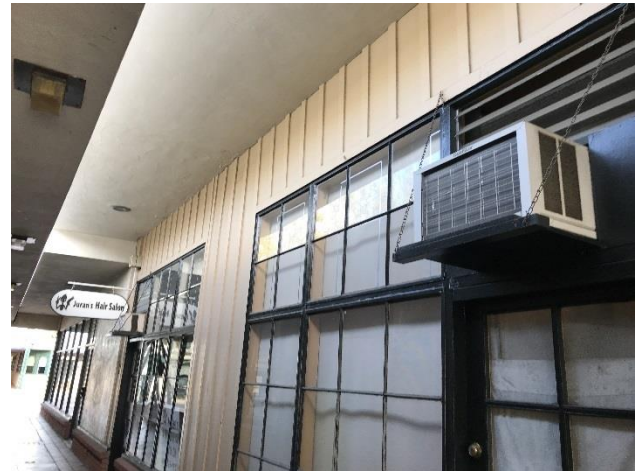
Above: Overdoor AC unit in breezeway.
