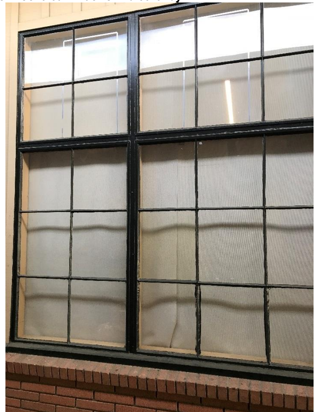
Below: Covered windows in breezeway.
