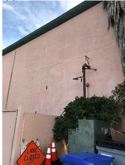
Below: Side façade with storage and mechanical equipment.
