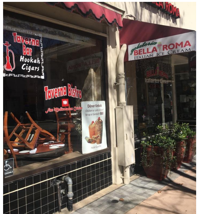
Above: Piping and conduit that distracts from the buildings architectural features.
