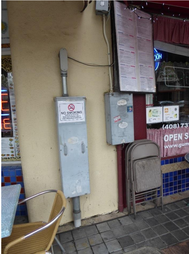
Above: Detail showing meters and conduit applied to exterior of building.
