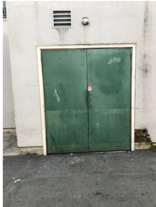
Above: Rear doors require repair and improvement.
