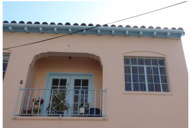
Below: Upper level balcony with railing and wood double doors and steel windows.
