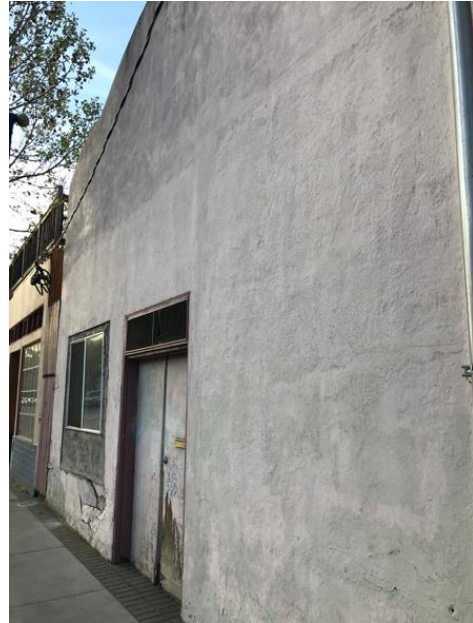
Above: View of required repairs to stucco, windows and doors at the Evelyn Avenue façade.
