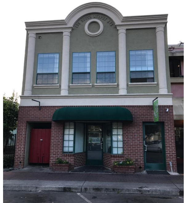
Above: Rear elevation with varying materials that do not provide a uniform or consistent appearance.
